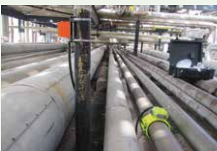
The iPerm system installed at Tüpraş facilities
